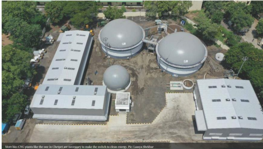
More bio-CNG plants like the one in Ghelpet are necessary to make the switch to clean energy. Pic: Laasya Shekhar
